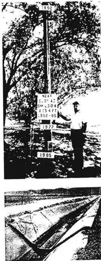
Figure 6. Subsidence broke and offset this irrigation canal in western Maricopa County. Photograph by L.D. Fellows.
